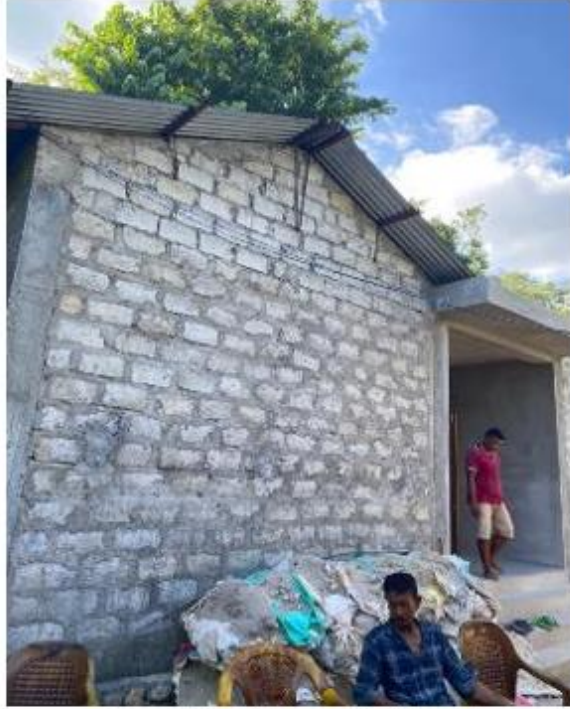
Incomplete HS house in Ghogrela
