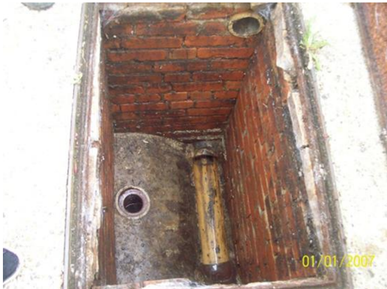
Figure 7. Dual manhole (London Borough of Harrow 2016).
