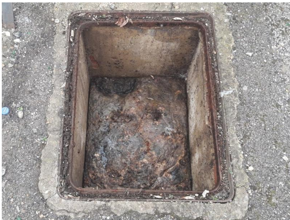
Figure 6. Blockage (Credit: Stephen Barry, Thames Water)
